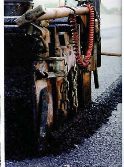
BELOW LEFT & BELOW: Volvo Construction Equipment's ABG8820 tracked pavers were used on China's Xian-Xun Highway BOTTOM: Temperature and sensor data from the MOBA's PAVE-IR Scan are integrated into the BPO Asphalt system
